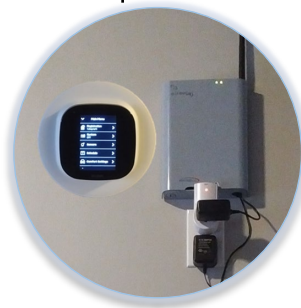
Smart thermostat & Wifi-enabled power meter
